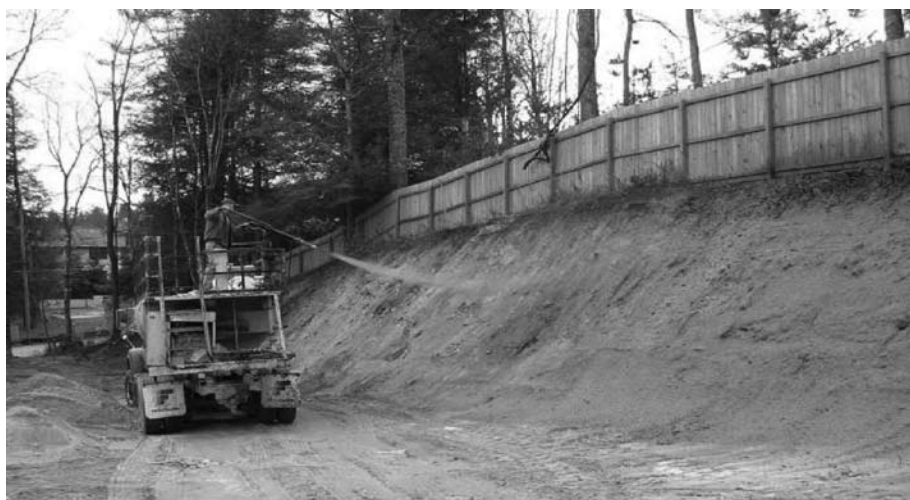
Figure 3. Seed, PAM, and a fiber mulch are applied to a steep slope with a hydroseeder.
