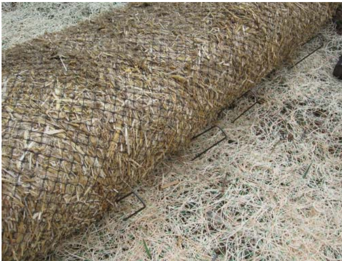
Figure 4. Example of how to install FCDs by stapling them to the ground through the netting on both sides. Staples have not been fully inserted into the soil in order to see their placement.
