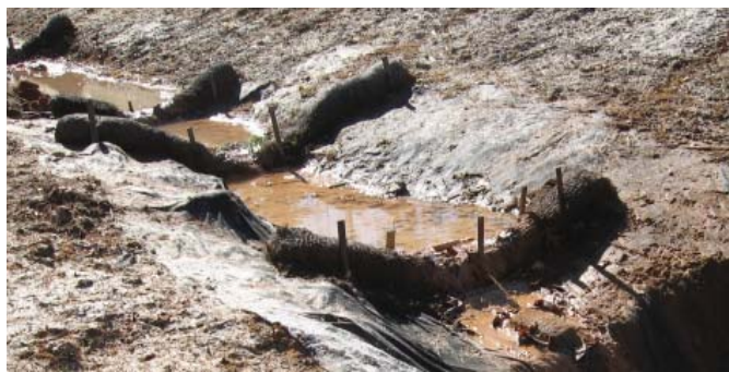
Figure 2. An example of an installed FCD system pooling water in a ditch line.
