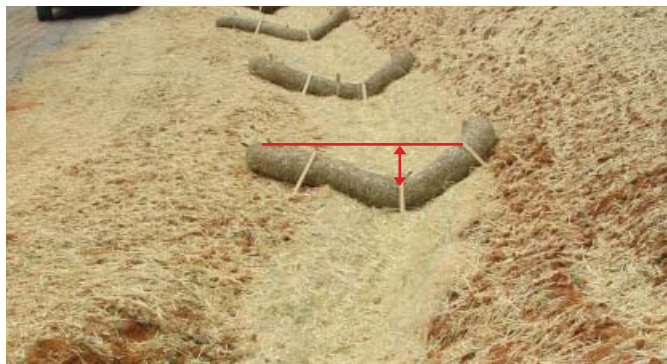
Figure 3. During installation, make sure that the FCD fits snugly into the ditch contour with no gaps and that there is clearly a lower, center weir section (the area denoted by the red arrow) set in the FCD large enough to withstand the storm event for which the ditch was designed.
