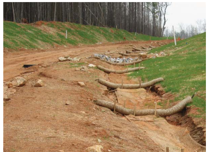
Figure 6. An example of improperly installed FCDs and ditch liner. The liner was not extended up the sides of the ditch, and the FCDs were not stapled into the ground. As a result, erosion occurred under the FCDs on the edges of the liner.
