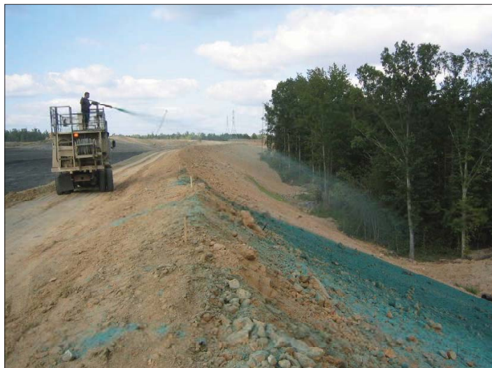
Figure 3. Hydromulching a large slope. This process should be repeated from the bottom of the slope. Note the berm at the top of the slope to prevent runoff from the upper areas from running onto the slope.
