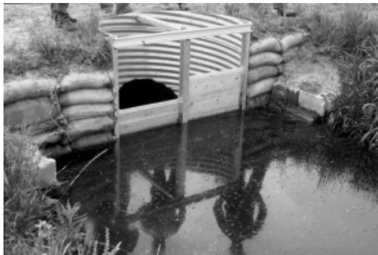
Figure 9a. Controlled drainage showing flashboard riser.
