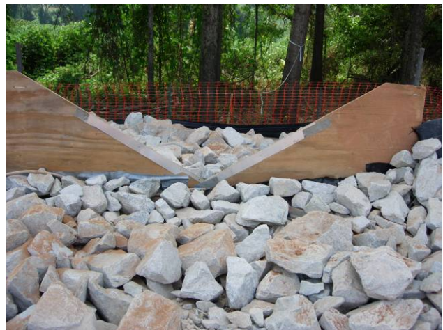
Figure 3. Weir used at Site WAKE2.
